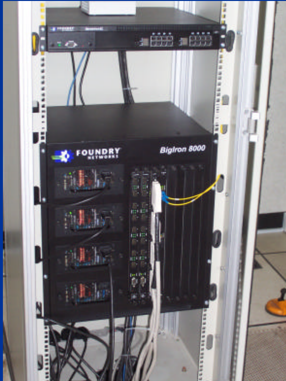
Equipment handling the Internet Exchange
